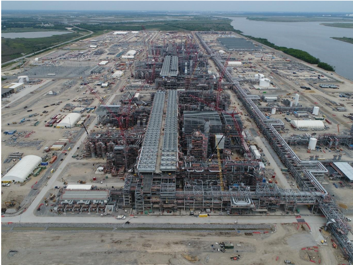
Overhead view of Train 1, May 2018
