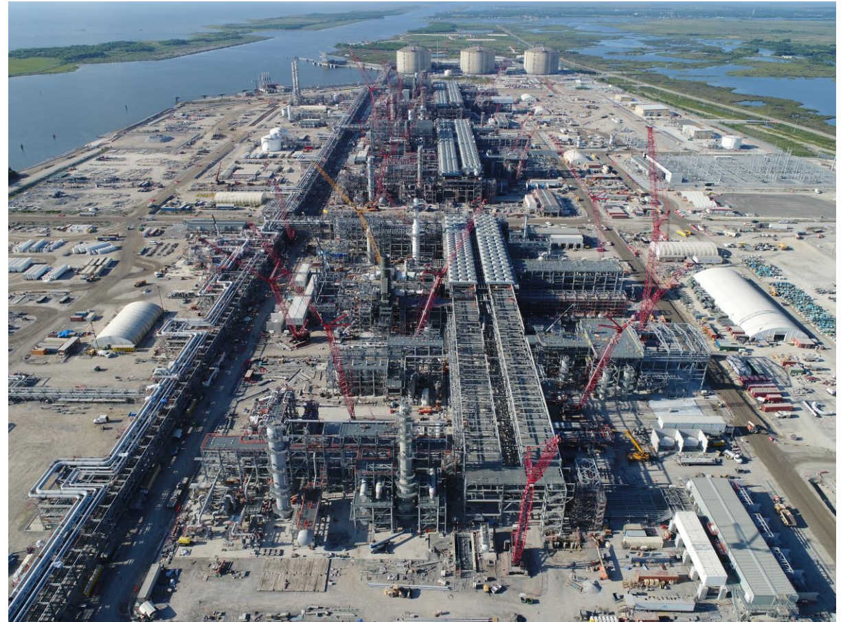
Overhead view of Train 3, May 2018
